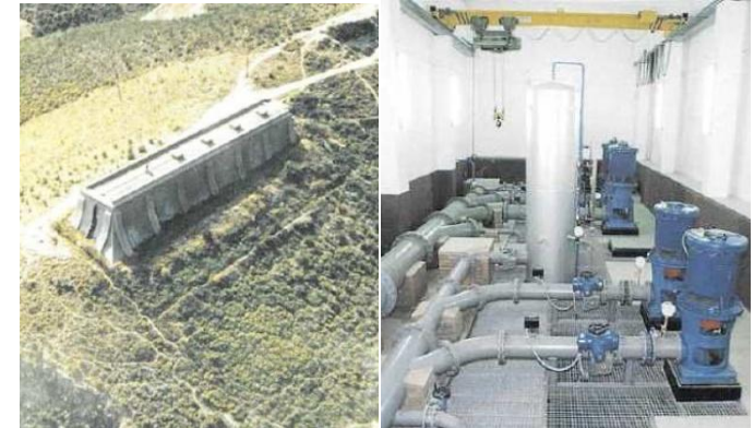
Tank and pumping station
