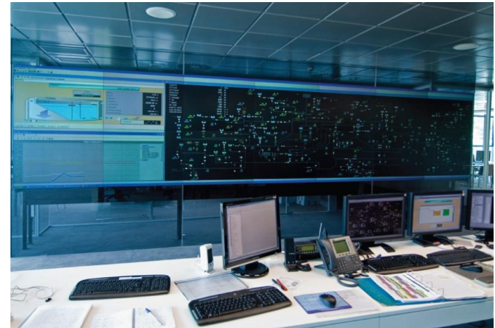
Water Network Control Center AGBAR Barcelona
